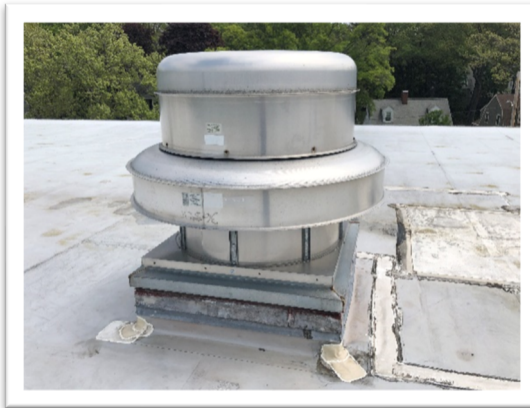
Photo 4: Exhaust Fan on 1949 Roof
