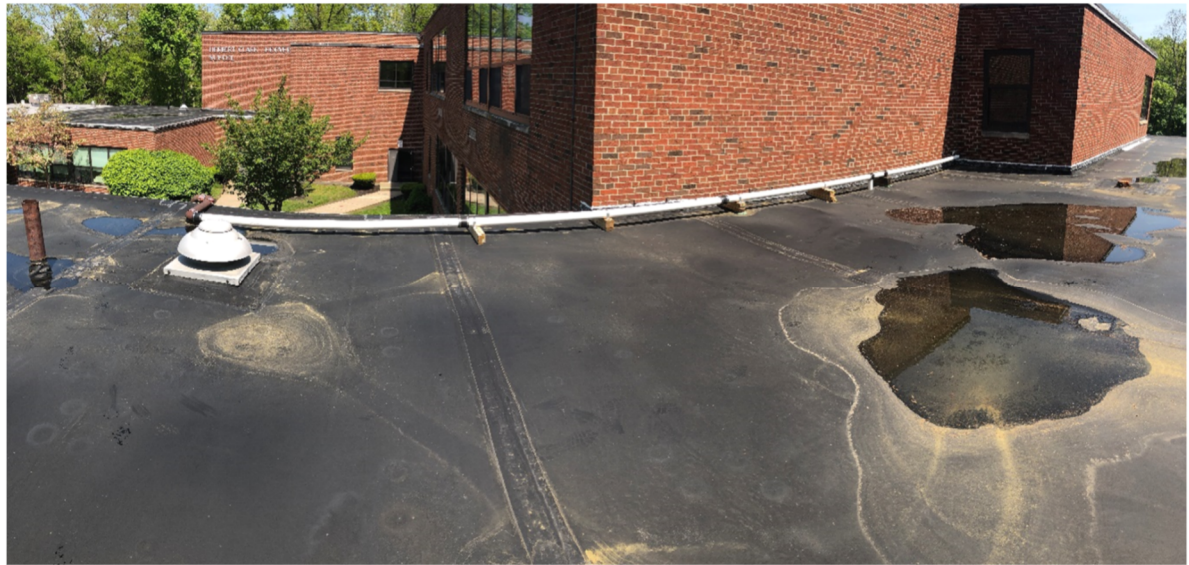
Photo 5: Storm Leader Routed on Roof
