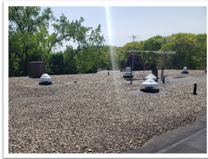
Photo 6: HVAC Equipment on Main Roof
