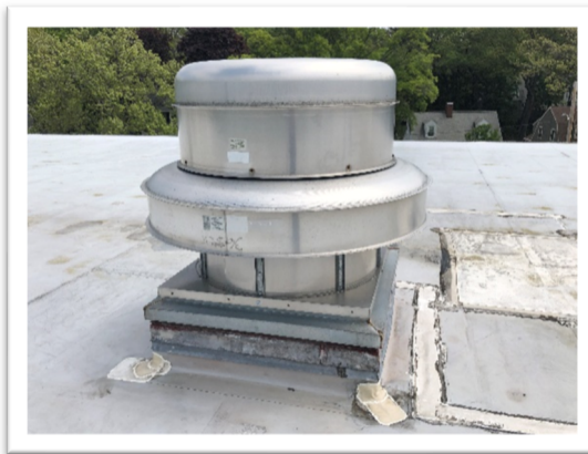
Photo 4: Exhaust Fan on 1949 Roof
