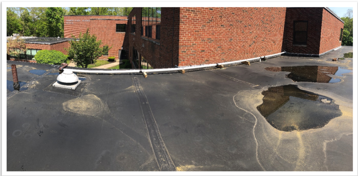
Photo 5: Storm Leader Routed on Roof
