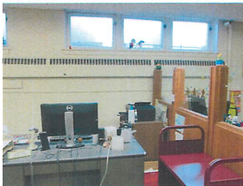
Technical services staff have very poor heating, as the radiators are above their heads, and emit a loud rattling noise throughout most of the day.
