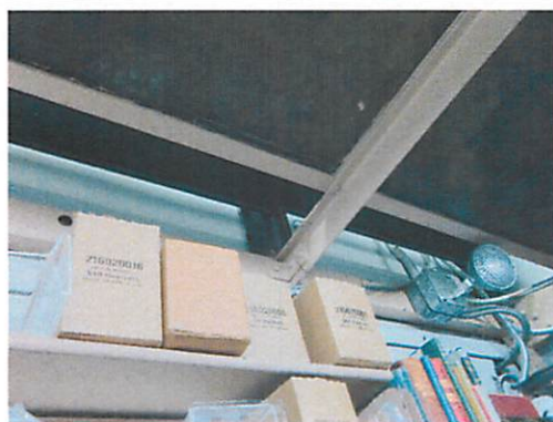
The ceiling is open to a public area, where debris is regularly dropped down onto office work. A memorable moment included digging a pebble out of the printer below!
