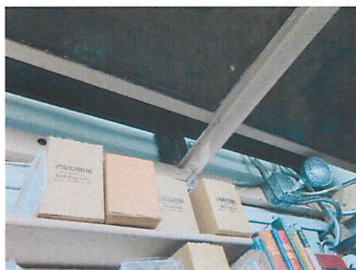
The ceiling is open to a public area, where debris is regularly dropped down onto office work. A memorable moment included digging a pebble out of the printer below!
