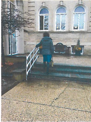
The main entrance has no ADA accessibility. It requires stairs, and there is no automatic door.
