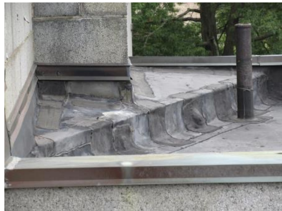
Image 90: Numerous patches were noted throughout the roof membranes on all roofs; this location on Roof Area E contained a particularly high number.
