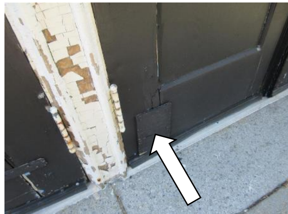
Image 70: Previous repairs (arrow) to the door leaves have become loose, and gaps were observed at multiple door leaves.
