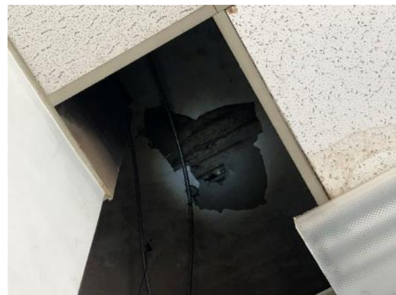
Image 10: Deteriorated plaster and lath ceiling above the suspended ceiling within the Kitchen
