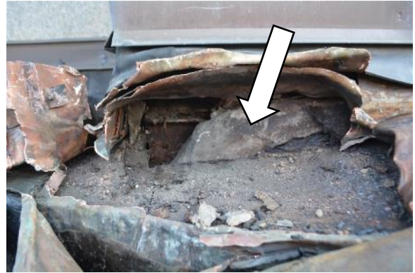
Image 12: Detail of the test cut showing the copper cladding and cementitious material (arrow) that coats the steel at this location
