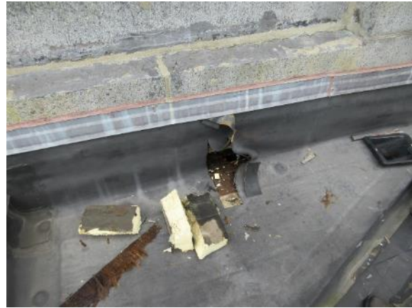
Image 100: Very wet plywood decking and corroded steel observed at Test Cut #14; refer to the Structural observations for more information.
