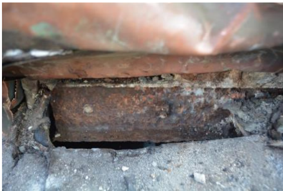
Image 11: The steel exposed at this location was found to be heavily rusted.
