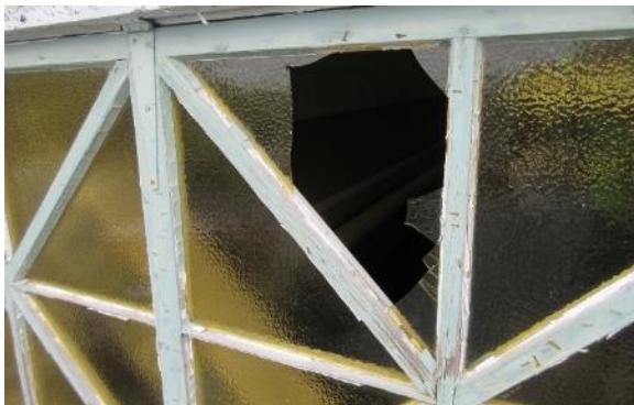
Image 53: Broken glass observed in the upper clerestory windows at the time of the evaluation.
