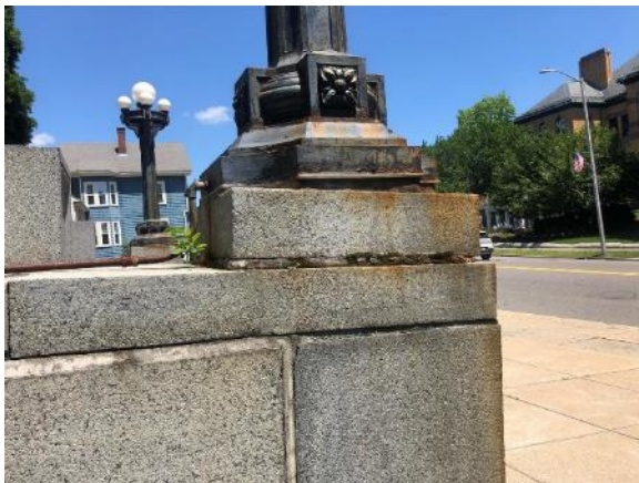
Image 127: The lamppost bases were stained and sit on a bed of deteriorated mortar.
