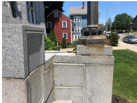
Image 128: The sloping of the entire stair structure can be observed below the lampposts, as the lampposts appeared to be installed plum, but sit on wedge-shaped grout bed on the sloping granite surface.
