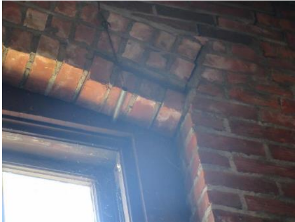
Image 11: Loose brick and delaminated mortar above the window in the rear storage room
