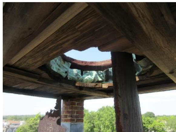
Image 116: Opening in the wood deck for the cast iron stack; the stack was found to be heavily rusted with portions missing.
