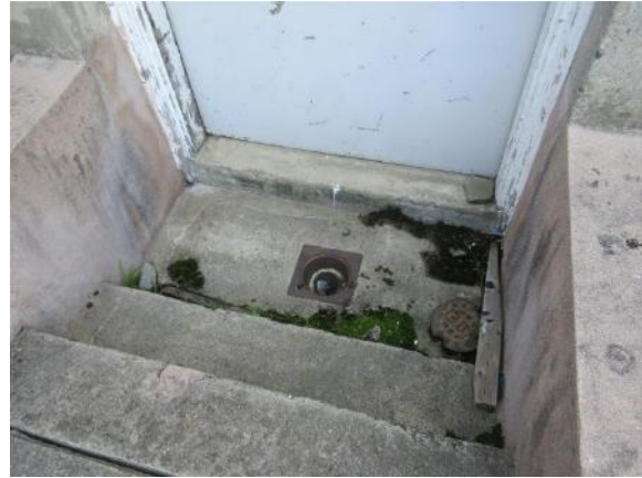
Image 84: Vegetative growth was observed on the landing in front of the door; a pipe possibly serving as a drain appeared to be clogged and non-functional
