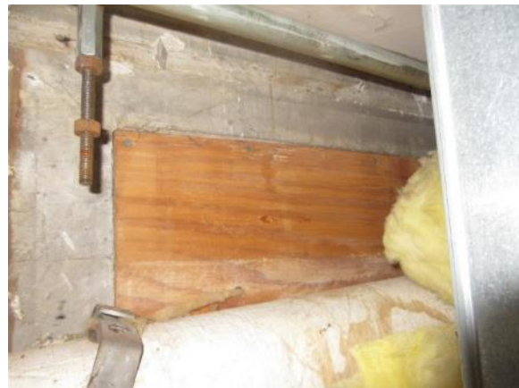
Image 50: Window concealed behind newer bathroom wall construction, also blanked-off on the interior with a plywood panel.
