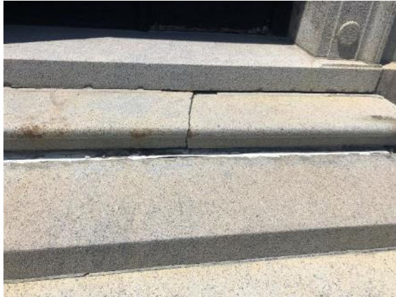
Image 129: A crack was found in the top-most stair tread in front of the door.
