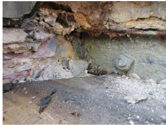
Image 12: The steel member was observed to be embedded in the parapet wall at the front of the building.
