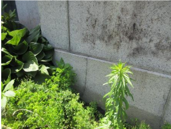
Image 17: Crack within a granite block at the front elevation near the foundation
