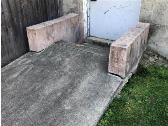
Image 83: Condition of the stair in front of the door; the concrete path leading to the stair is beginning to separate from the stair structure; erosion of the fill beneath stair was noted
