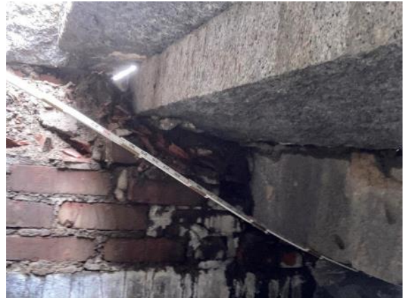
Image 122: View within the cavity looking towards a brick pier that supports the larger middle stair treads. Brick and mortar at this location was found to be loose and crumbled.
