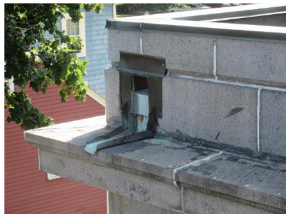
Image 112: Drainage from Roof Areas D and E are provided by scuppers that drain onto Roof Areas F and G; no downspouts are installed at these locations
