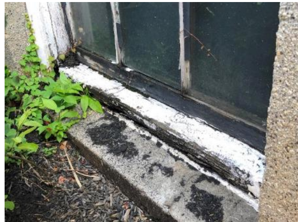
Image 44: Heavily deteriorated sill and window components at a rear basement window.
