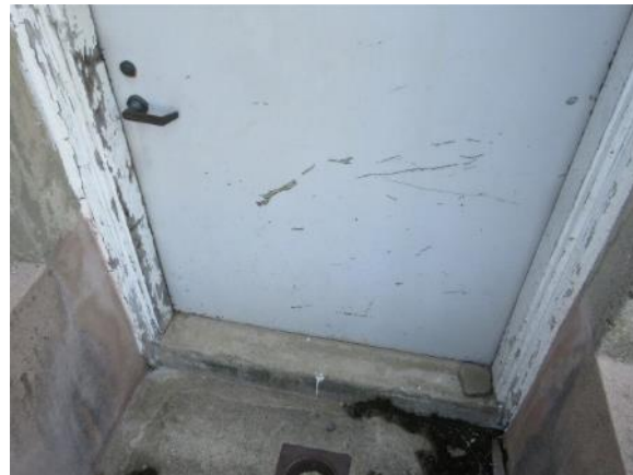
Image 82: Detail of the door trim and leaf exhibiting flaking and crazing paint and scratches in the paint on the door leaf.
