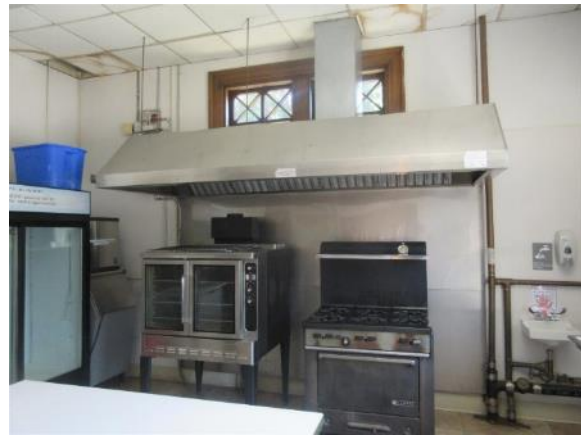
Image 48: The vent hood blocks access to a window within the kitchen; the hood is visible from the exterior.
