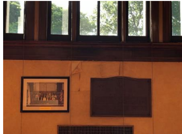
Image 2: Peeling wallpaper below front window sills
