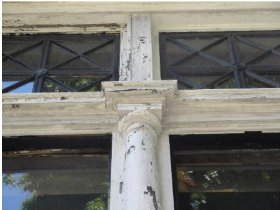
Image 41: Detail of a column capital as part of the window framing for Window Type D. Flaking paint is typical for all windows.
