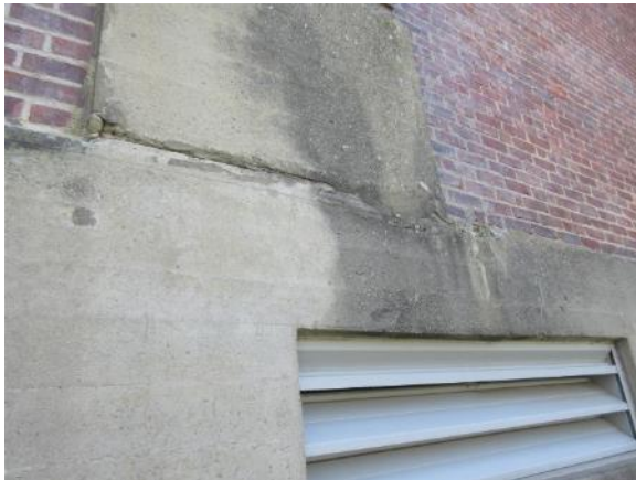
Image 29: Spalling and cracking in the concrete at the Addition
