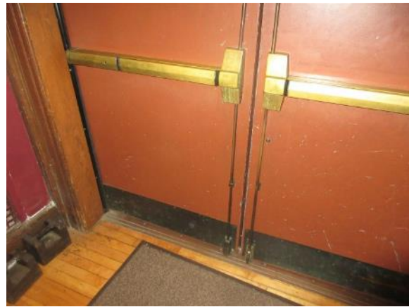
Image 74: Scratches in the paint were observed on the door leaves.
