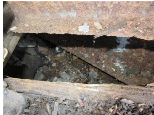
Image 12: The steel member was found to be supported on a diagonal steel member similar to Roof Area D.
