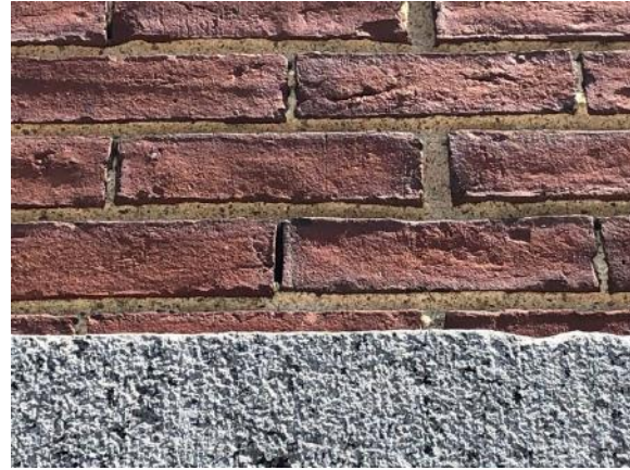
Image 26: Typical deteriorated and missing mortar joints at the brick inset areas at the original building
