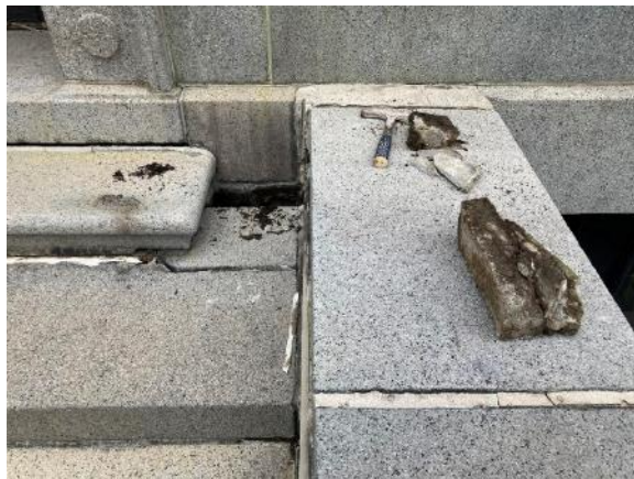
Image 123: A portion of grout was also removed at the large joint between the stair structure and the building.
