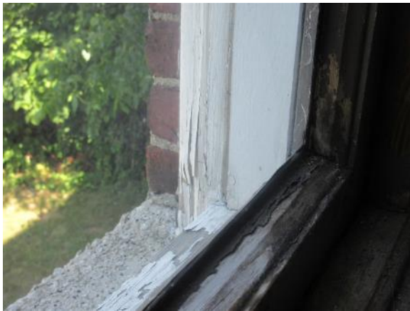
Image 47: Degraded interior paint and finishes on the windows and sills were noted at some locations.
