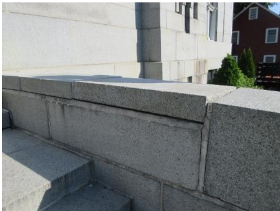
Image 125: Wing wall cap stones were found to be displaced with open mortar joints.
