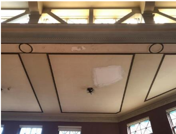
Image 7: Peeling paint and previous plaster repairs on the Auditorium ceiling
