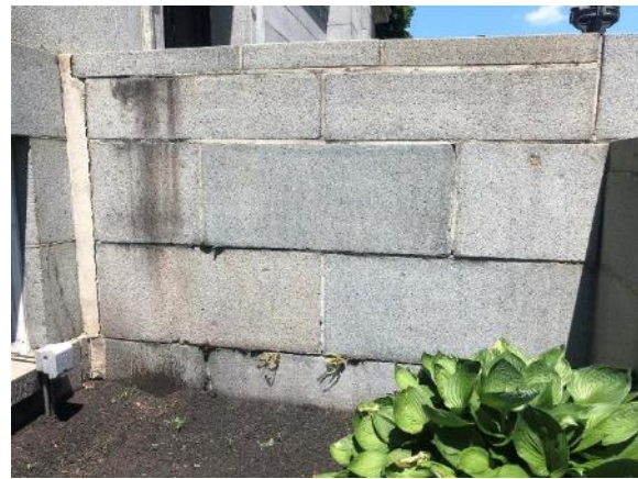
Image 126: Vegetative growth and open mortar joints were observed on the sides of the wing walls.
