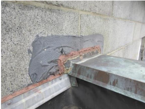
Image 105: Deficient termination of the parapet cap flashing on Roof Area C that is sealant-dependent
