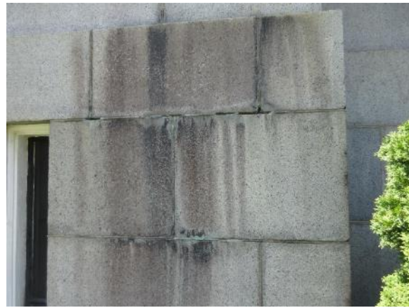
Image 16: Typical staining and deteriorated mortar within the granite at the front elevation
