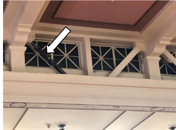
Image 6: Missing finishes on trusswork within the Auditorium
