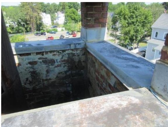
Image 115: The tops of brick walls below the cap are flashed with lead-coated copper flashing that appeared in fair condition.
