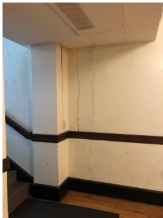
Image 3: Cracks in plaster within the basement immediately below the GAR Hall
