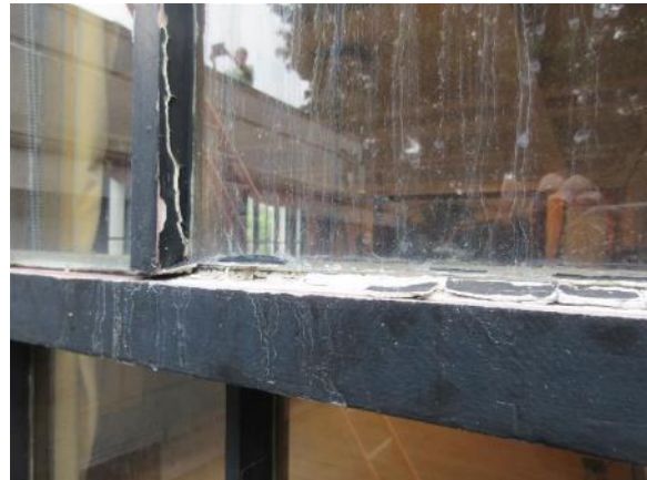
Image 42: Typical deteriorated glazing putty between the glass and the sash frame.
