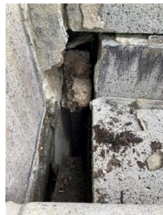
Image 124: The grout material was found to crumble upon sounding. A wood element was observed at this location and appeared to be displaced from its original position.
