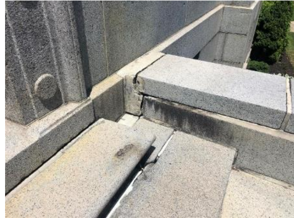
Image 130: Gaps observed in the joints between the stair structure and building.
