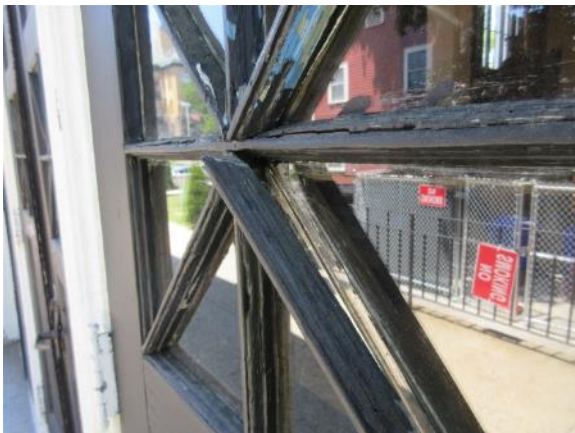
Image 69: Loose muntins and deteriorated glazing putty was noted throughout all of the doors.
