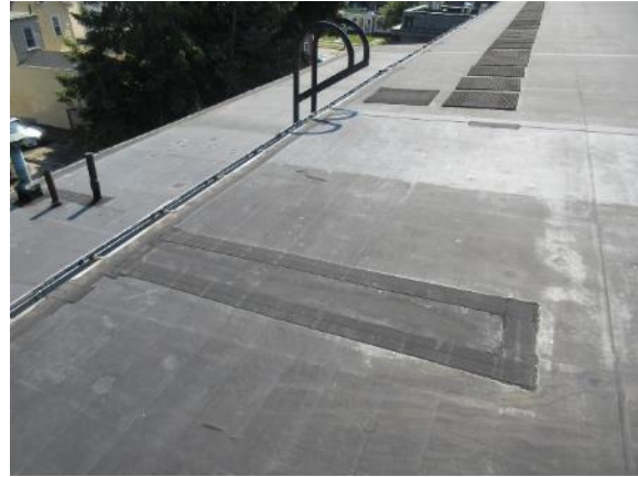
Image 92: Large patches with deteriorated seams were noted in numerous locations.
