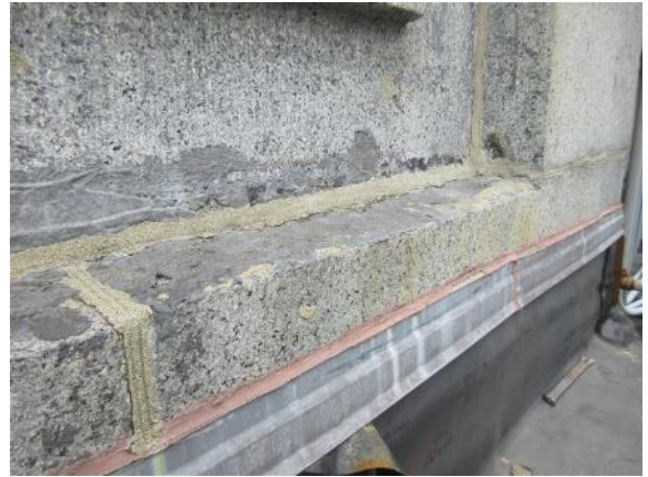
Image 106: Exposed ledge at inset area above Roof Area C without flashing or protection; roof-to-wall flashing detail utilizes a surface-mounted reglet flashing whose sealant was found to be deteriorated.
