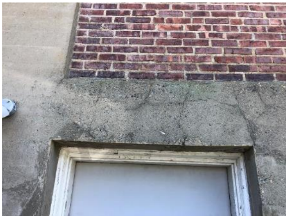
Image 31: Network of small cracks above the basement door at the Addition
