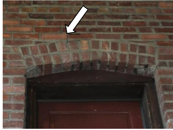
Image 12: Step crack (arrow) above organ access door in the rear storage room
