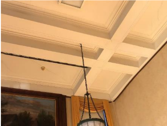
Image 5: Area of general plaster cracking in the GAR Hall ceiling (area is above Image 3)
