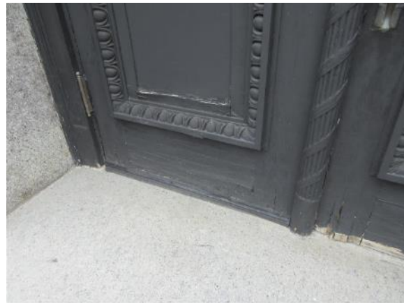
Image 64: Deteriorated wood elements noted at the base of the door leaves
