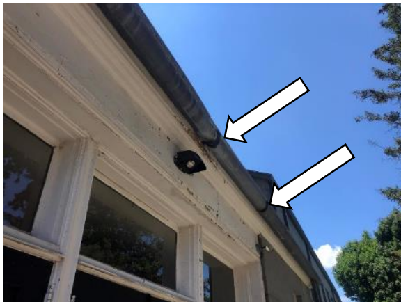
Image 109: Additional active gutter leak locations that have been attempted to be sealed with duct tape (arrows)
