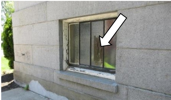
Image 51: Broken glazing covered with tape (arrow) at the basement window on the North Elevation
