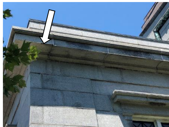
Image 22: Spalled ledge stone (arrow), as well as staining on the ledges and previous sealant repairs at the mortar joints
