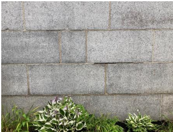
Image 15: Typical mortar condition within the granite; patchwork of missing mortar and mortar repairs
