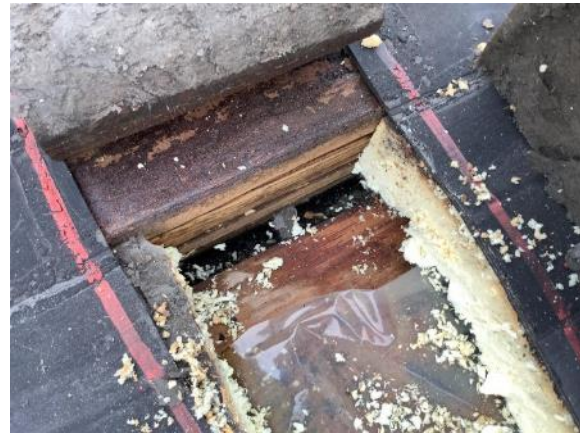
Image 96: Water staining observed on the roof deck at Test Cut #5.
