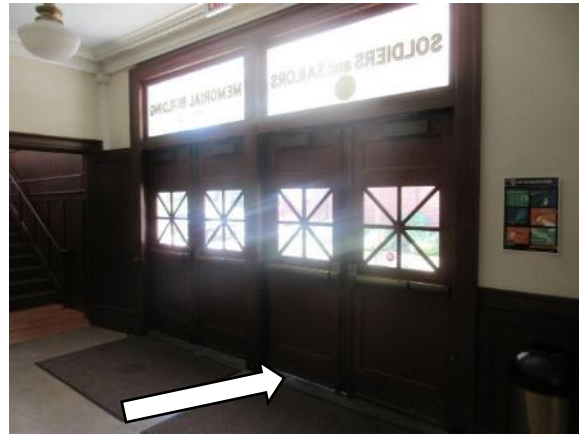
Image 80: Interior of the main entrance doors; daylight was observed coming from beneath one of the doors (arrow).
