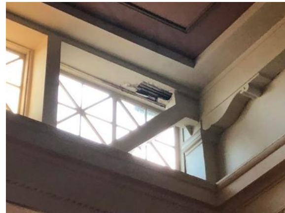
Image 8: Missing portions of plaster finishes at the upper clerestory windows
