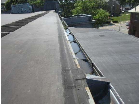
Image 107: Standing water observed in the gutter on the south side of Roof Area A at the time of the evaluation
