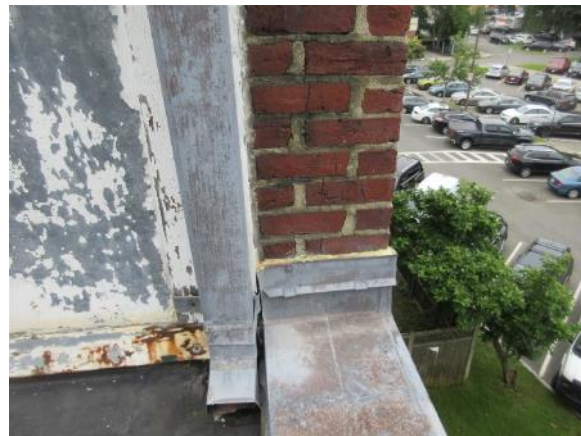
Image 24: Cracked brick and deteriorated mortar the brick parapet rising walls
