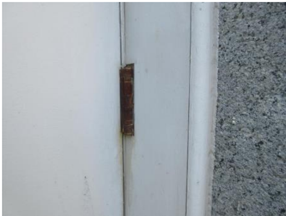
Image 73: Hinges at the doors were exposed to the exterior and were found to be rusted.
