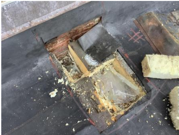
Image 95: Crumpled and unterminated vapor retarder at Test Cut #3.
