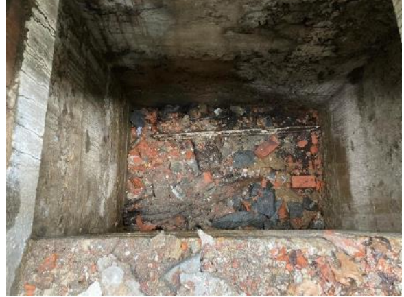
Image 120: Removal of the stair revealed an open cavity below that is filled with rubble and debris.
