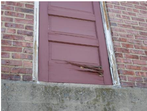
Image 77: Large chunks of the wood in the panels were found to be loose; the exterior brick moulding was found to be fraying and opening up.
