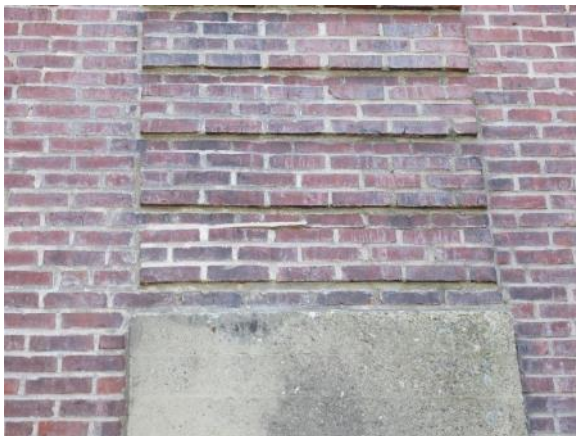
Image 27: Deterioration of mortar wash above the brick quoins
