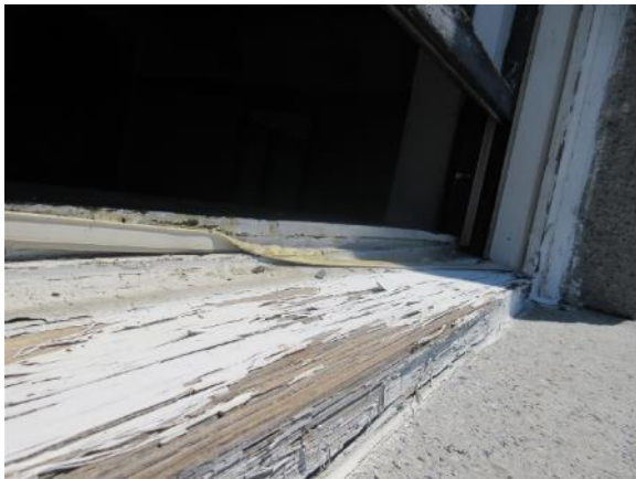
Image 43: Heavily deteriorated sills were noted at the windows with the 2 nd story changing room on the south side of the building.
