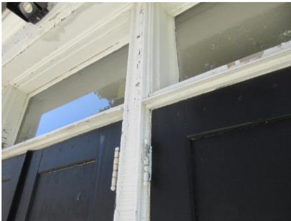
Image 67: Typical condition of the wood frame and trim with flaking and crazing paint observed throughout.
