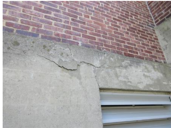
Image 30: Large crack above a louver at the Addition
