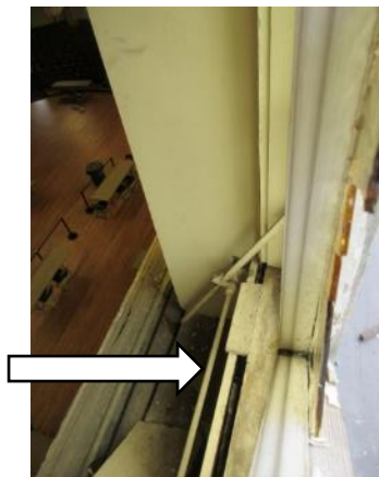
Image 59: Operating hardware for the awning windows at the upper clerestory windows, utilizing a crankshaft (arrow) operated from behind the stage
