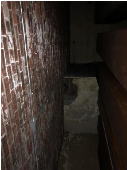
Image 13: Staining on plaster ceiling where the roof meets the rear brick wall
