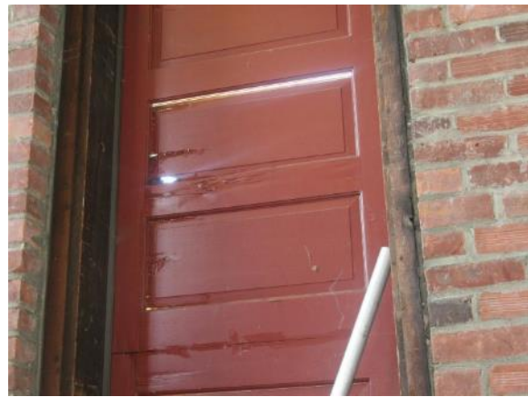
Image 78: Wood in the door panels was found to heavily deteriorated throughout, and gaps were observed in the door panels.
