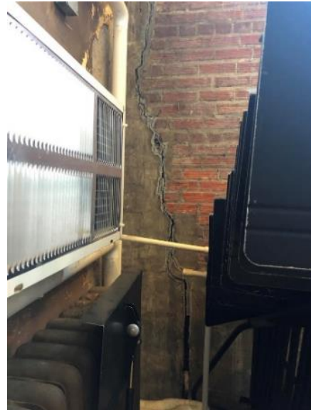
Image 14: Crack at the expansion joint at the Addition within the rear storage room
