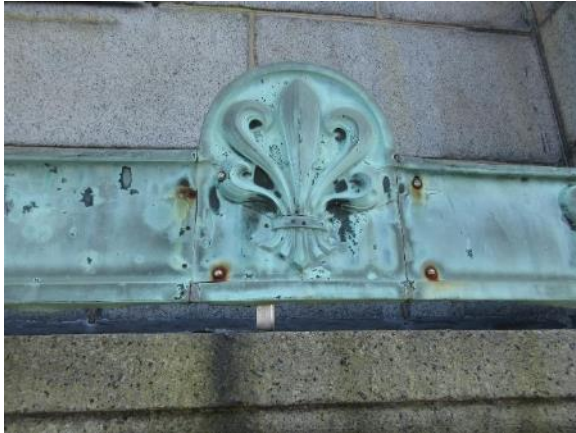
Image 39: Detail of a typical pendant in the horizontal banding. Rust was noted around fastener locations. Pitting and staining on the brass was observed throughout the banding.
