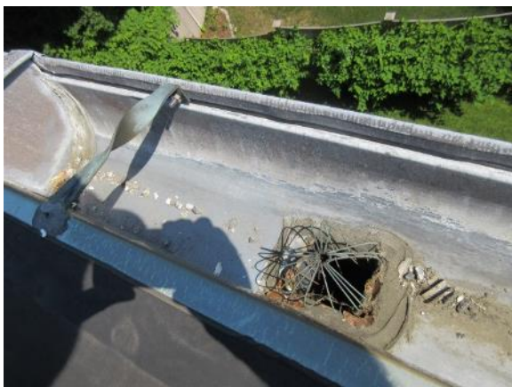
Image 111: Downspout strainers were found to be deflected and, in some cases, displaced from the downspout opening.
