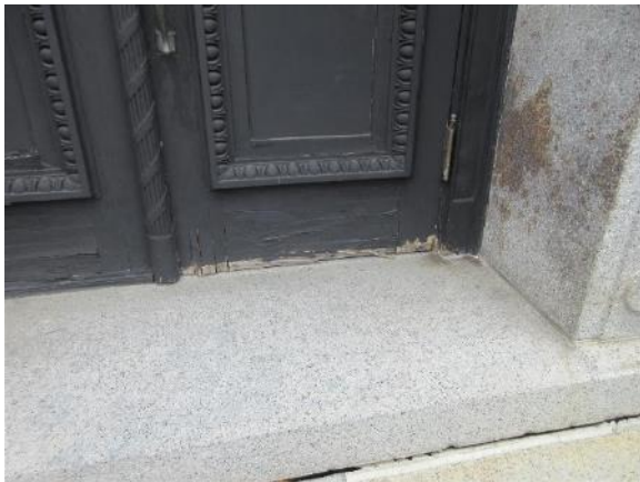
Image 63: Missing door sweep at one of the door leaves
