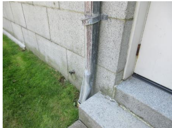
Image 110: The majority of the downspouts were found to be deflected at their lower portion near grade
