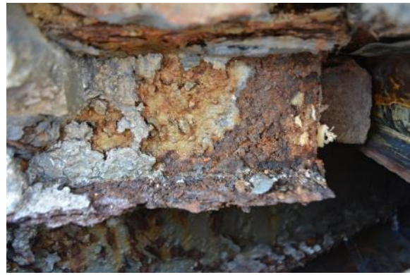
Image 12: The steel immediately below the masonry wall exhibited heavy rusting and portions flaking away
