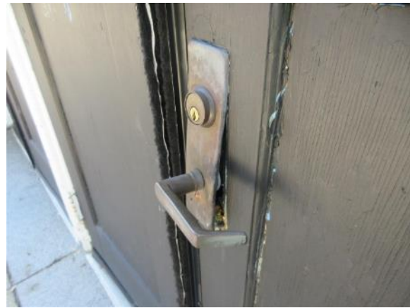
Image 68: Displaced and loose door handle was noted at one of the door leaves
