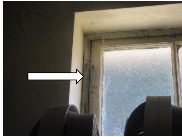
Image 60: Chain (arrow) for the operation of the basement hopper windows; arrow indicates a broken chain.
