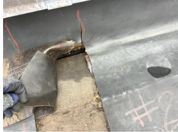
Image 94: Wet insulation observed at Test Cut #2.
