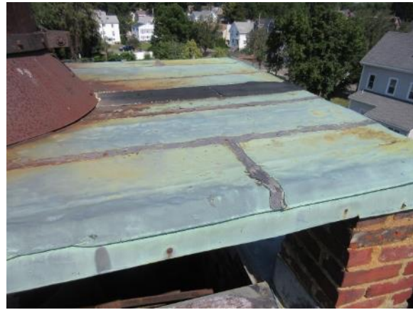
Image 114: Flat-seam copper panels were found to be pitted and deflected with seams repaired with sealant.
