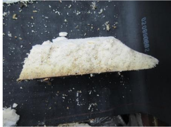
Image 98: Staining was observed in the top portion of the insulation at most test cut locations
