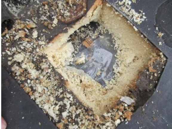
Image 93: The plastic vapor retarder was not terminated at all perimeter test cut locations.
