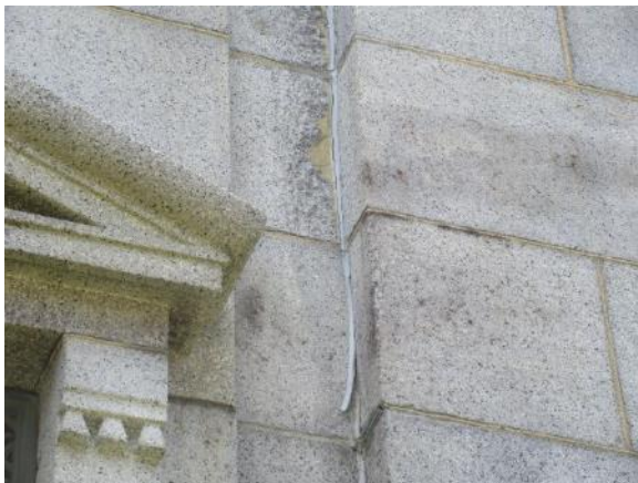
Image 19: Failed sealant around the perimeter of a recess in the granite facade
