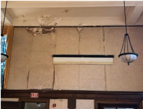
Image 1: Significantly peeling wallpaper and paint in the GAR Hall
