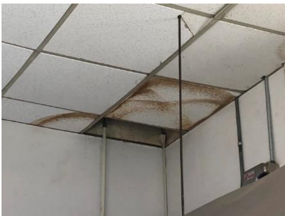
Image 9: Typical water staining on the ceiling tiles within the Kitchen
