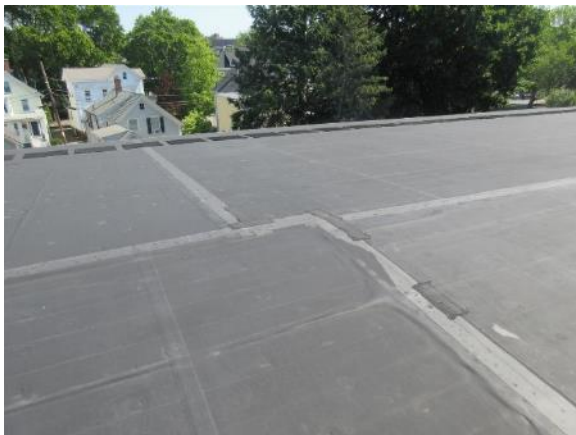
Image 89: Deteriorated seams were noted throughout the roof membranes on all roofs
