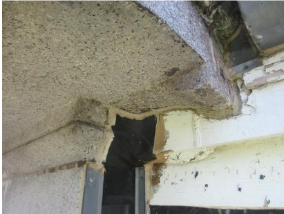
Image 103: Sealant-dependent flashing configurations at the upper clerestory rising wall to granite wall transitions.
